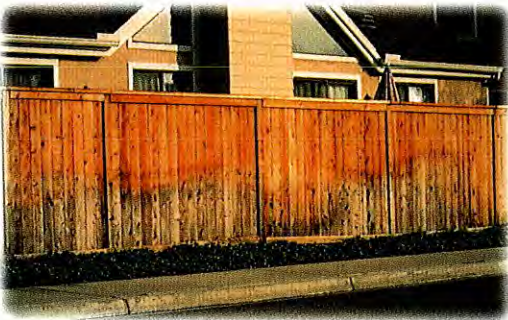
(Top) Old fence with water damage. (Above) New fence with water damage.
