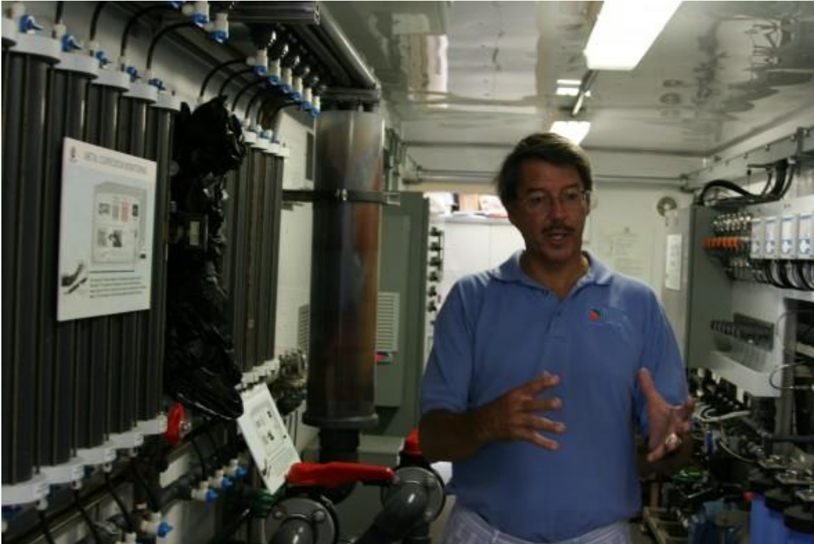
Inside Doheny Beach pilot desal plant
