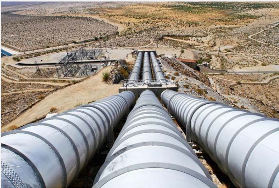
The Julian Hinds Pumping Plant is one of the hydraulic hearts of California's vast water supply system, built to push water from where it is to where it isn't, no matter how many hundreds of miles of desert, mountains and valleys are in the way. (Irfan Khan, Los Angeles Times / September 8, 2011)
